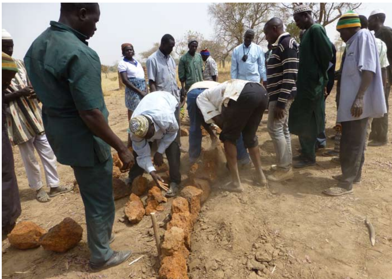
Farmers learning to construct rock barriers on contour to conserve soil and water.
